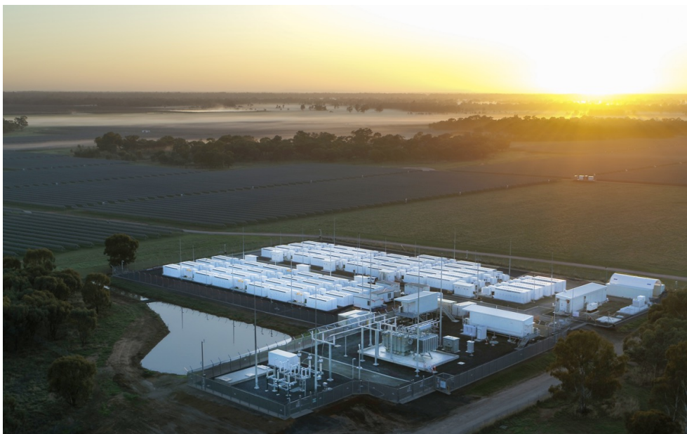
Federation's Riverina Battery Energy Storage System
